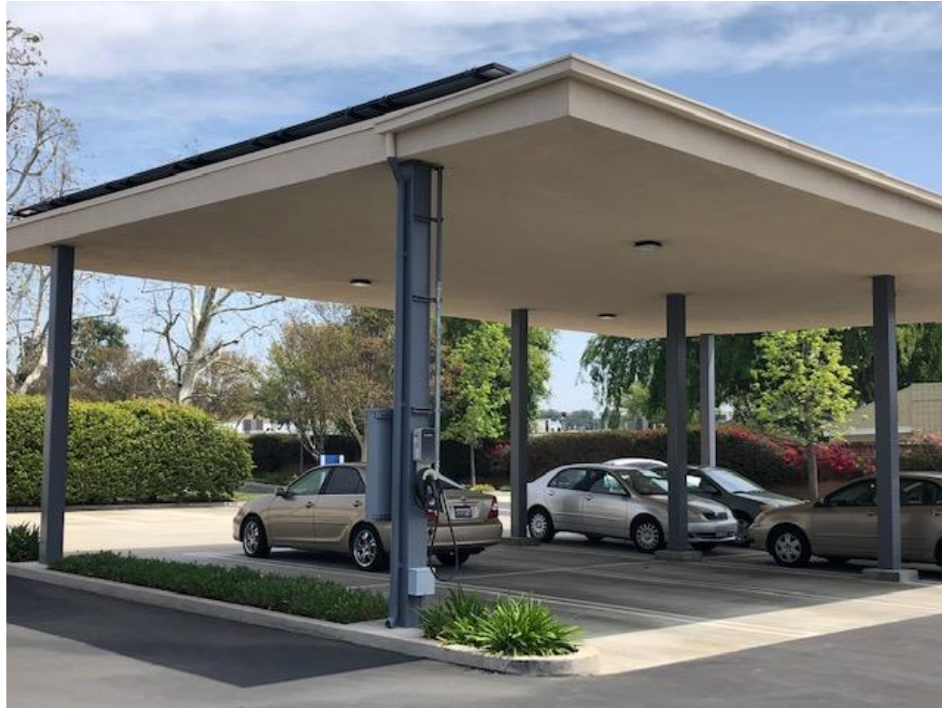
Carport with solar panels (on top) and electric vehicle recharging station
